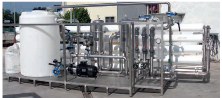
Ultrafiltration and Reverse Osmosis Recovery System
